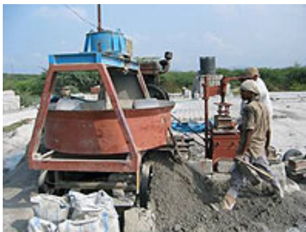
10 workers working in a plant produce about 2 million bricks per year on single shift operation
