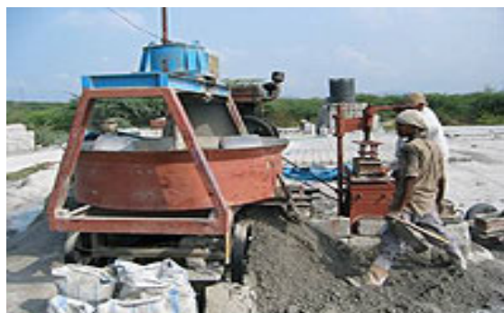
10 workers working in a FaL-G plant producing 2 million bricks/year on single shift operation
